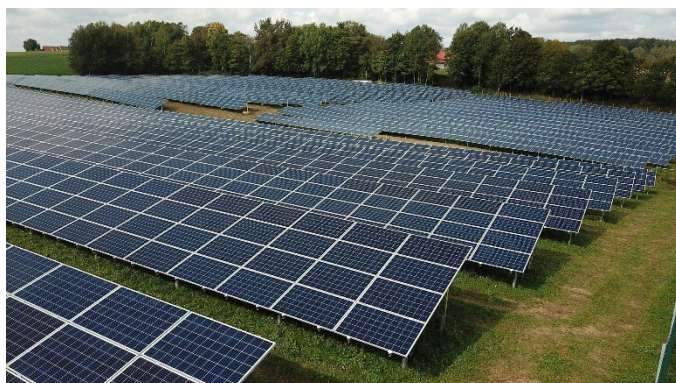
Figure 1: A photo of a Community Solar Energy System (Source: ysgsolar.com)
